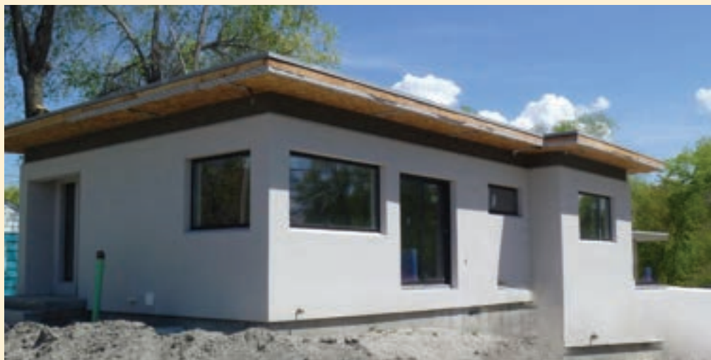
The "Emery House" will include 2,100 square feet, 4 bedrooms, 2.5 bathrooms and a two car garage when it is completed in June. The mid-century modern house is designed to be very energy efficient and will be certified through the Passive House Institute US ( www.phius.org ).
